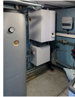
PAC air/eau Atlantic Excellia + Centrale solaire photovoltaïque
