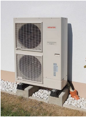
PAC air/eau Atlantic Excellia + Centrale solaire photovoltaïque
